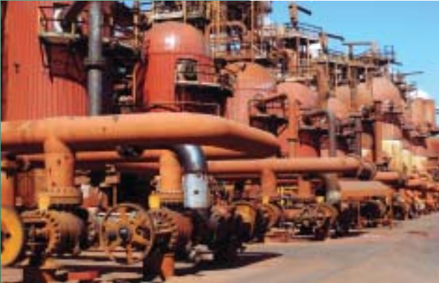
Scale build-up costs the alumina industry millions annually. (Photo courtesy of QAL)
